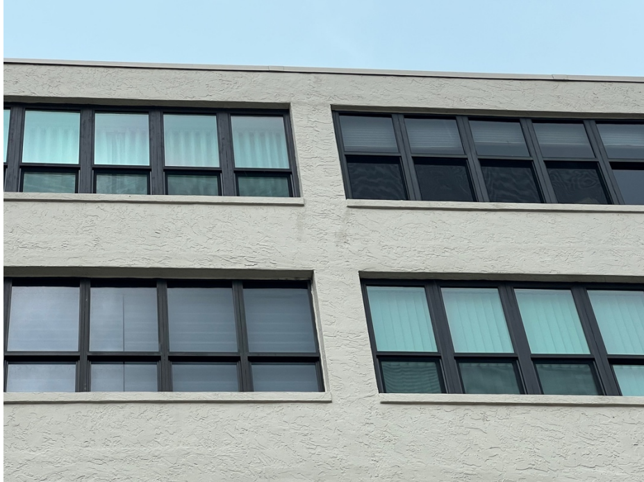
Example of East elevation (facing the Ritz) showing inconsistency of replacement windows including window manufacturers, color, material, opening size, and glass tint. This is meant as an illustration only, reinforcing the need for a consistent standard.
