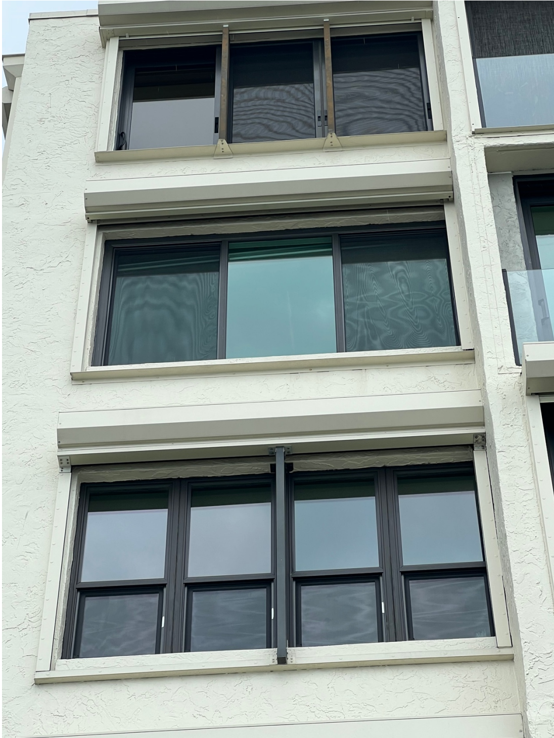
Example of West elevation (facing LBK) showing replacement window inconsistency in window type and opening ranging from sliding and casement (non-original) to double hung (original). This is meant as an illustration only, reinforcing the need for a consistent standard.
